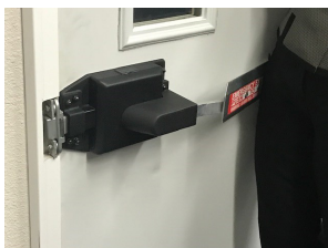
Isolation room door with bar lock that requires a person to lean against to engage.
