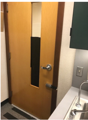
An isolation room with a substantial part of the window covered by black paper, obstructing the student's view outside the room.
