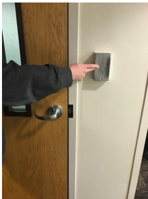
Isolation room door lock that requires a magnet to engage.
